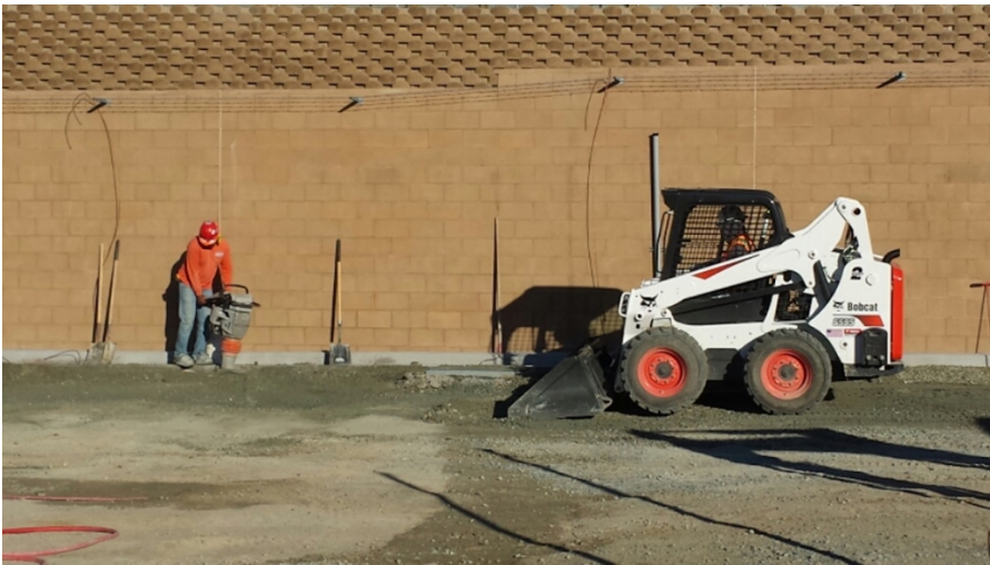
Photograph 2: Grading and installing base within the substation occurred during the week of March 11, 2017.
