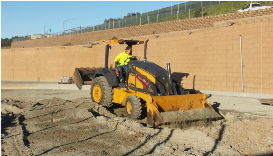
Photograph 1: Grading within the substation occurred the week of March 18, 2017. All ground disturbances was in previously disturbed fill.
