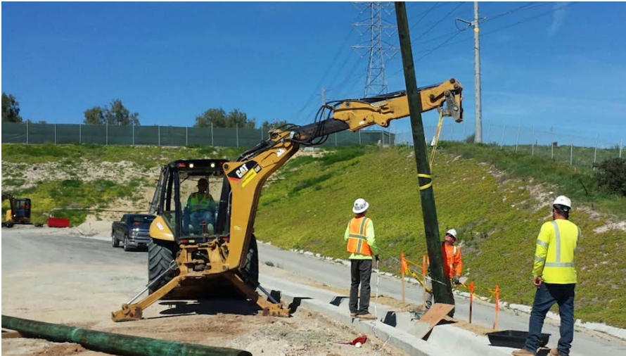
Photograph 1: Installing poles for temporary power to the substation occurred the week of March 11, 2017.
