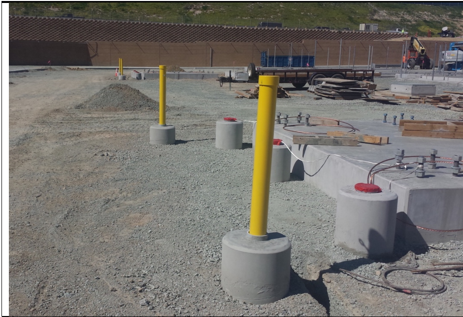
Photograph 3: Paint and primer applied to bollards in the substation were found to exceed Project limits on VOCs resulting in a Level 3: Compliance Issue on March 8, 2017.
