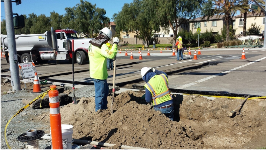
Photograph 3: Pot-holing to locate irrigation lines in Exploration Falls driveway occurred the week of March 04, 2017.
