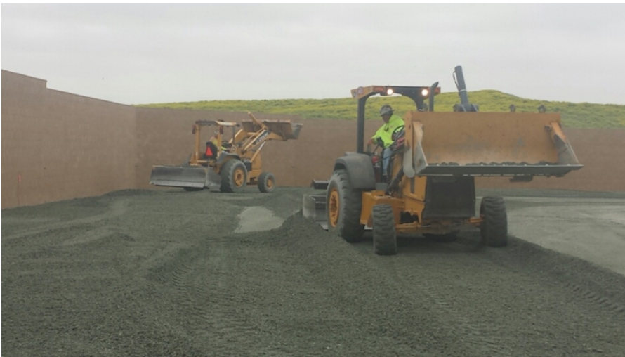
Photograph 2: Installation of Class II base in the battery storage yard occurred during the week of March 25, 2017.
