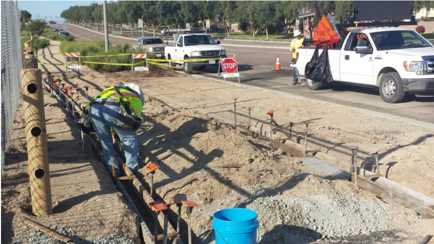
Photograph 1: Pedestrian ramp and mow strip installation at the Exploration Falls Dr. driveway occurred the week of March 25, 2017.
