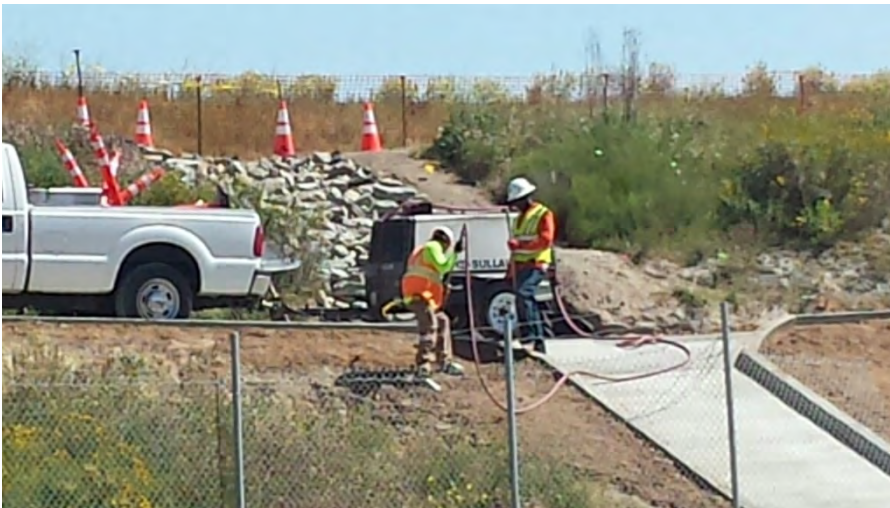
Photograph 2: Arizona crossing and spillway installation on the corridor road occurred during the week of April 8, 2017, 2017.
