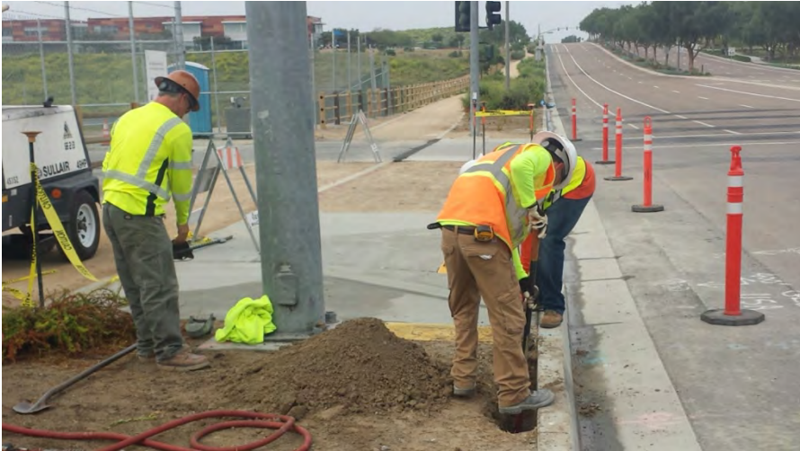
Photograph 1: Landscaping irrigation repairs at the Exploration Falls Dr. driveway occurred the week of April 8, 2017.
