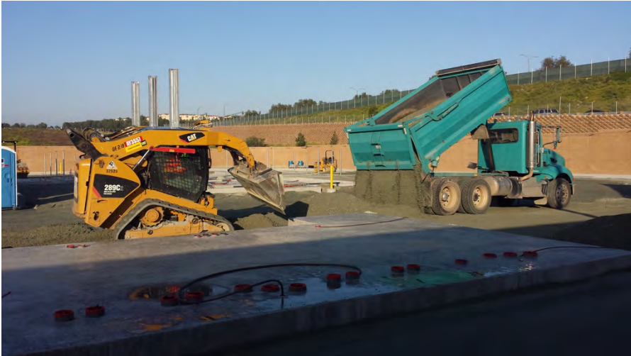
Photograph 1: Import and installation of Class II base in the substation occurred the week of April 15, 2017.
