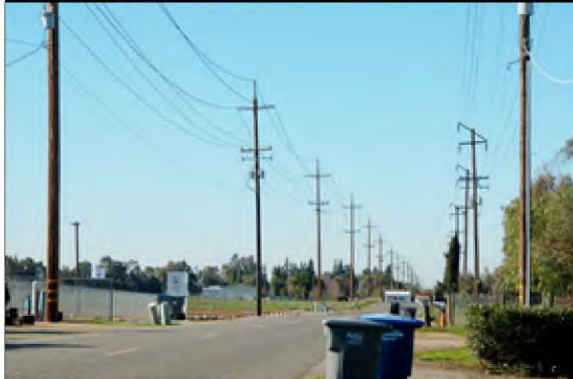
Photo #13: View looking west from E. Copper Avenue to existing power lines. Date of photograph: January 11, 2011.
