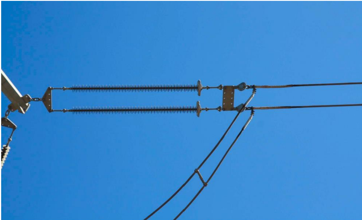
Figure 2.2-15 Representative Photograph of Bundled Conductor
