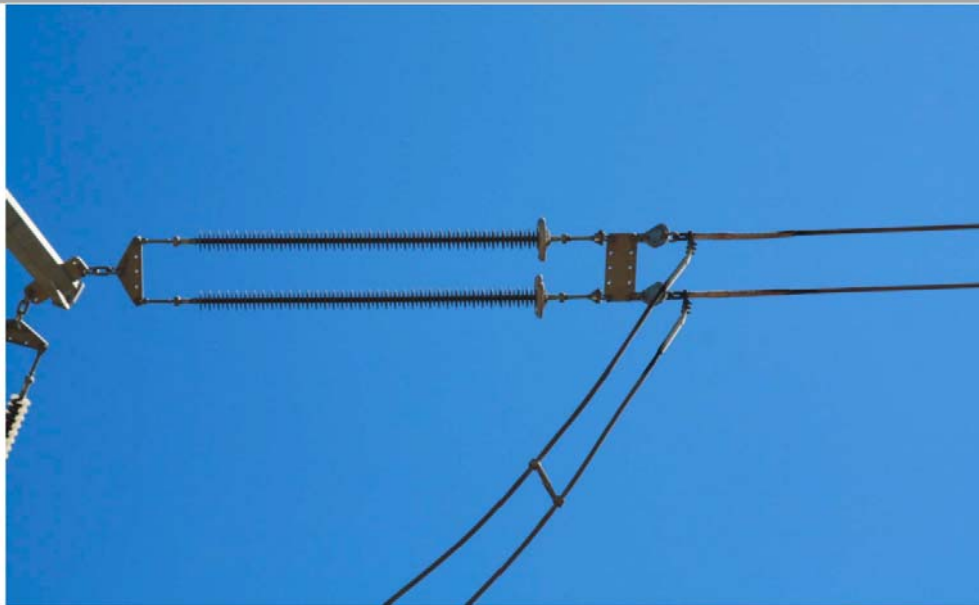
Figure 2.3-3: Representative Photograph of Bundled Conductor
