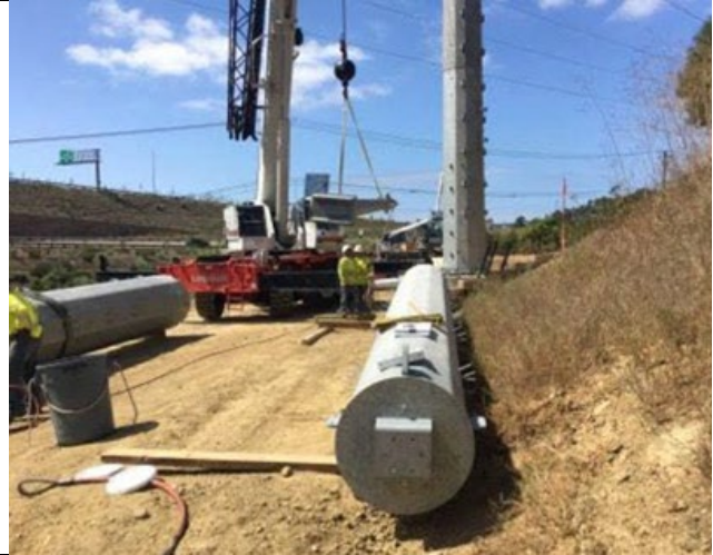
2: Assembling a steel pole; the pole was delivered in pieces and assembled on site
