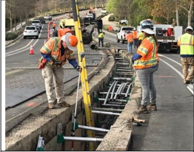
1: Trench to install conduit for conductor. One lane of traffic is open on the left side of the photo
