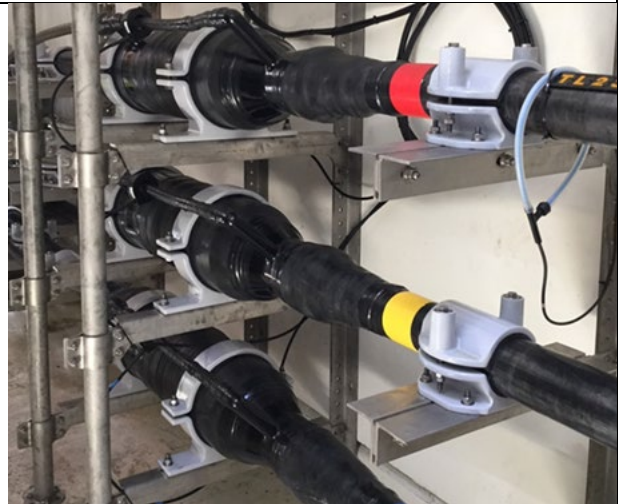
4: Conductor on racks inside of a vault
