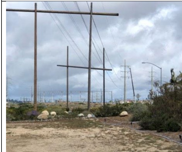
3: Guard structures were used to protect roads and other overhead power lines during conductor stringing; a crane is visible in the background conducting work on the steel pole
