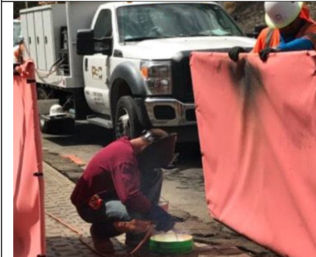
3: Welding together trench plates to cover the open trench; fire blankets are used to contain sparks
