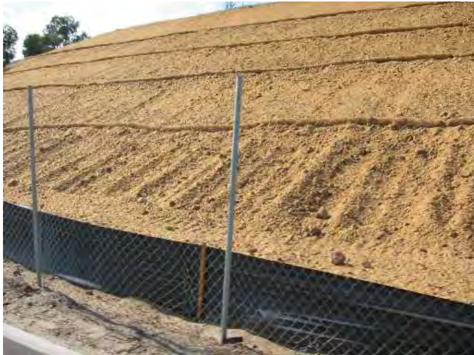
Silt fence installed with at least a 3 foot setback from the toe of an erodible slope. Note that use is combined with fiber rolls and serves as perimeter control.
