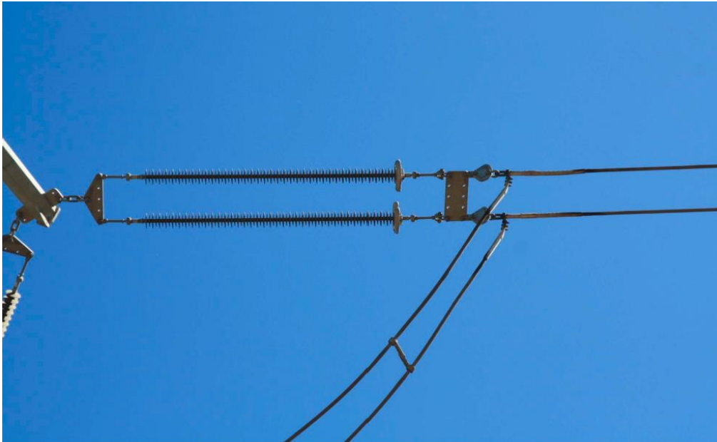
Figure 2.2-15 Representative Photograph of Bundled Conductor
