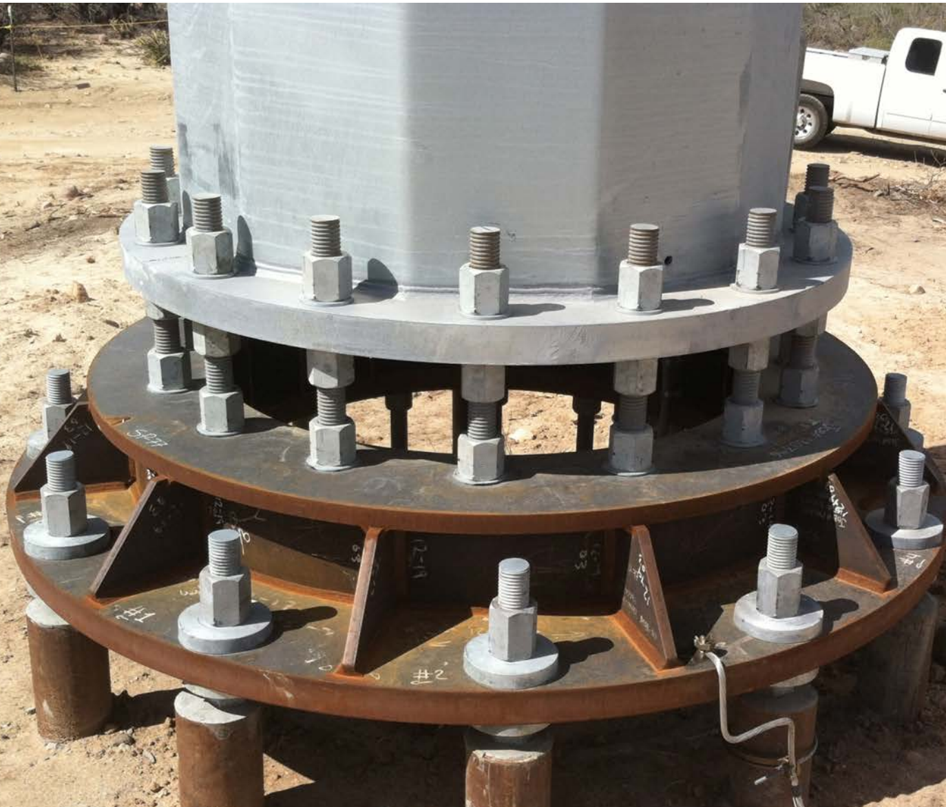
Typical 230kV Micropile Foundation with Anchor Bolts *Note that transition plate and micropile casing(s) would be galvanized steel similar to tubular steel pole coating.
