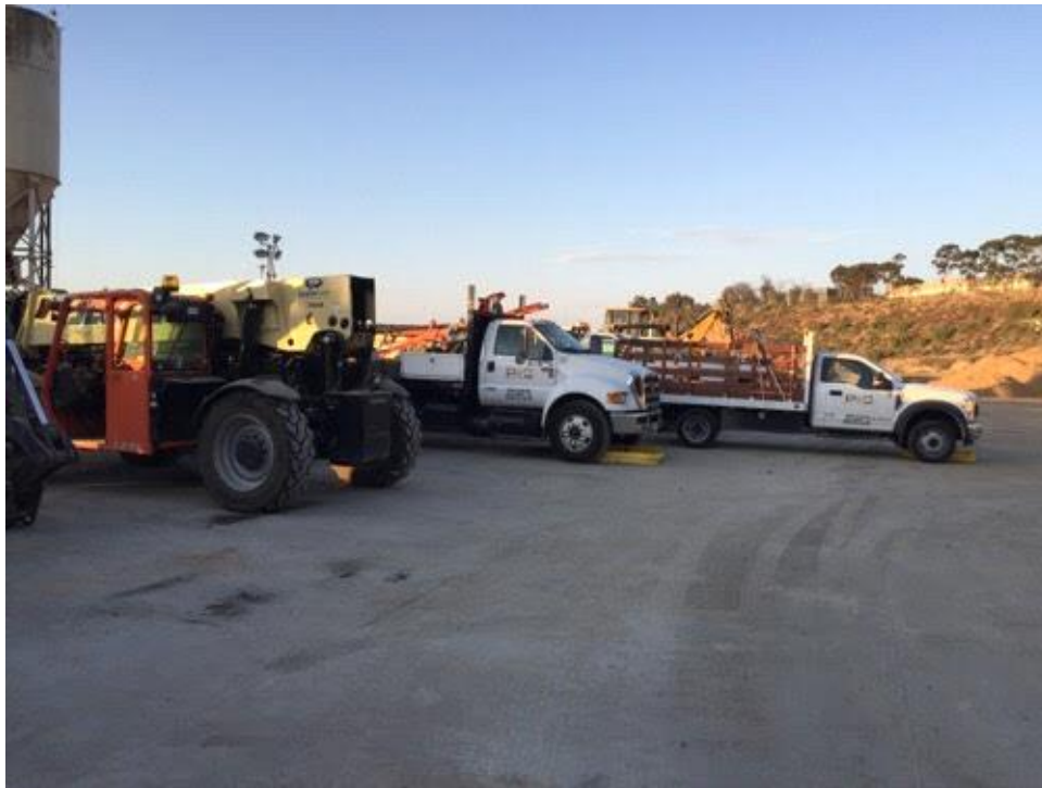
Caption Drip pans in place at construction yard off of Santa Fe.
