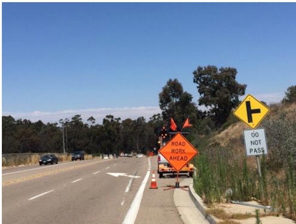
Caption Signage in place on Pomerado Road.
