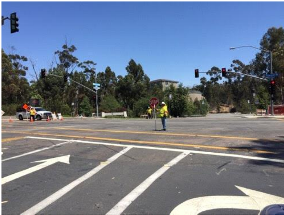
Caption Traffic flaggers in place on Pomerado Road and Willow Creek Road.
