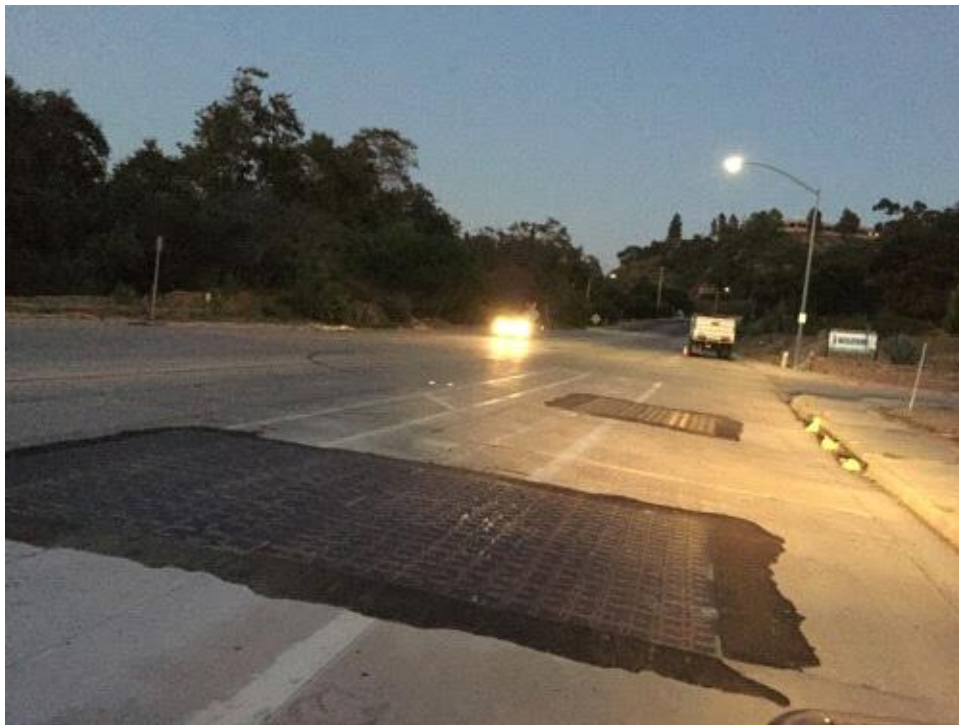
Caption Steel plates covering excavations when not in use on Carroll Canyon Road.
