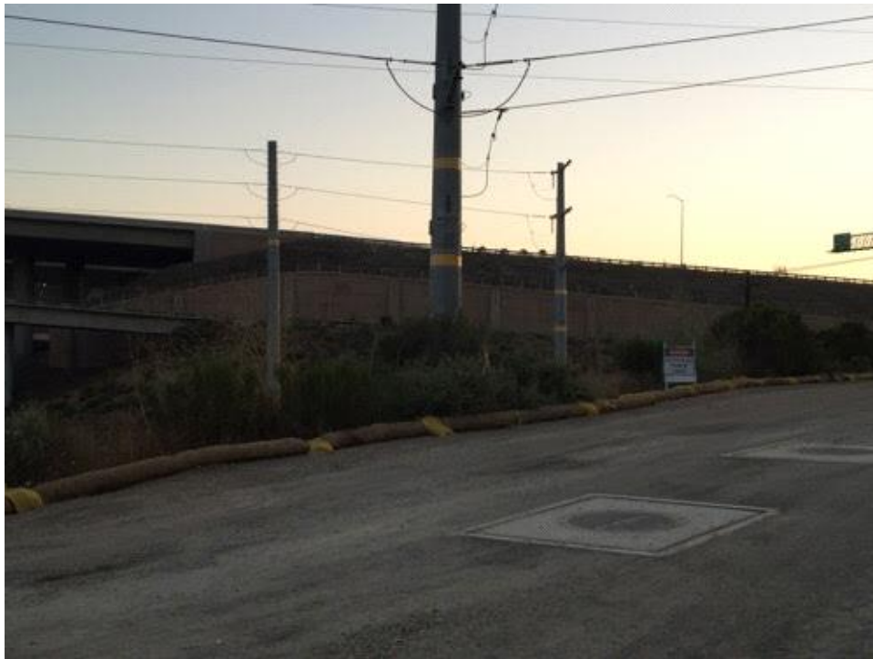
Caption BMPs in place and in good working order on Carroll Road near the 805 freeway.
