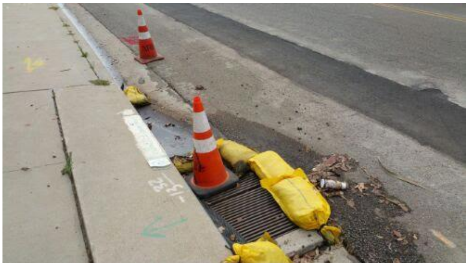
Caption Sediment detention at storm drain inlet (Trade St.).
