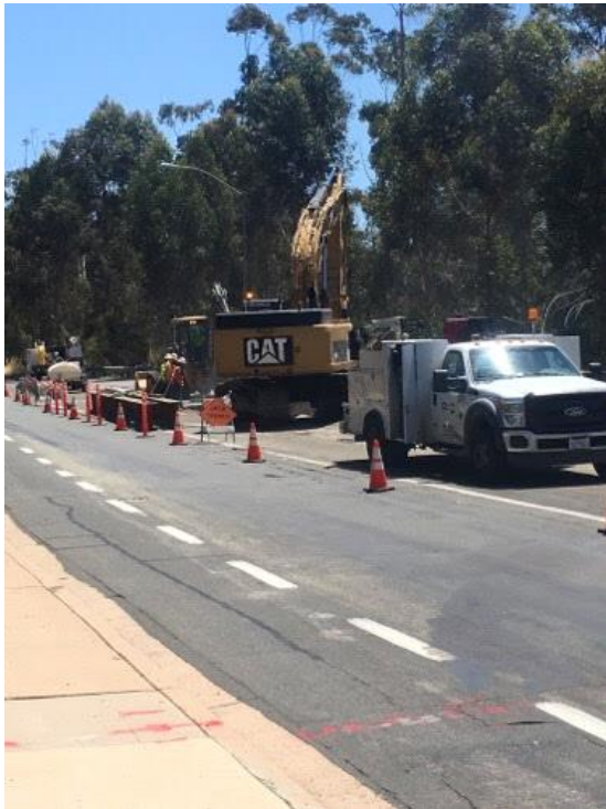
Caption Excavation on Pomerado Road. Photo Attributes Capture Date/Time: Tue Jul 11 2017 11:40:21 GMT-0700 (PDT) Coordinates: 32.897826, -117.102354 View Direction: East
