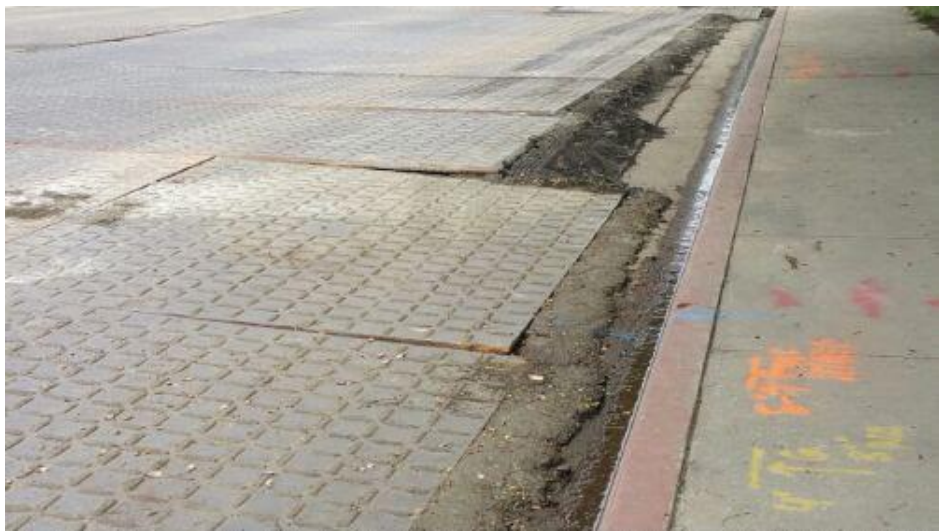
Caption Loose plate placement (Trade St.).
