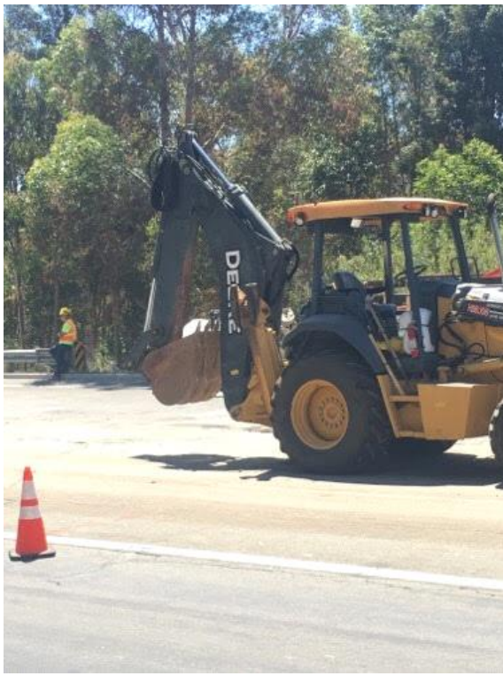
Caption Fire tools and fire technician onsite at Pomerado Road vault excavation. Photo Attributes Capture Date/Time: Tue Jul 11 2017 11:40:51 GMT-0700 (PDT) Coordinates: 32.897831, -117.102360 View Direction: Southeast
