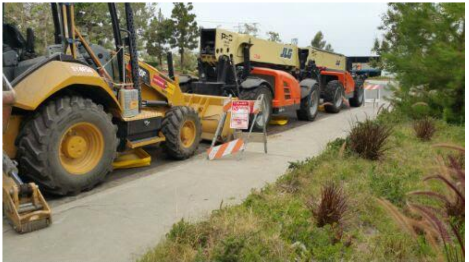
Caption Drip pans beneath equipment off Carroll Rd.
