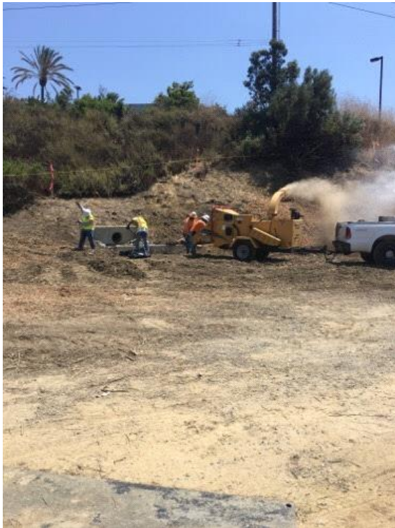
Caption Mulching at CCCMP Photo Attributes Capture Date/Time: Mon Jul 10 2017 11:31:18 GMT-0700 (PDT) Coordinates: 33.134508, -117.190868 View Direction: North
