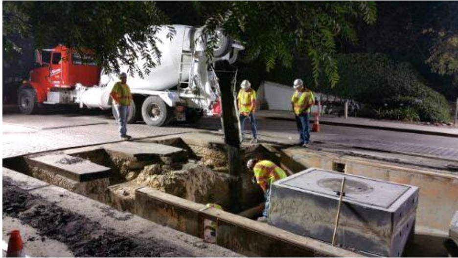
Caption Concrete pour into vault (Trade St.). Photo Attributes Capture Date/Time: Thu Jul 13 2017 21:15:18 GMT-0700 (PDT) Coordinates: 32.888781, -117.165494 View Direction: South
