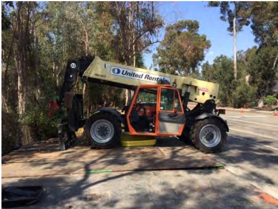
Caption Drip pans in place on Pomerado Road.
