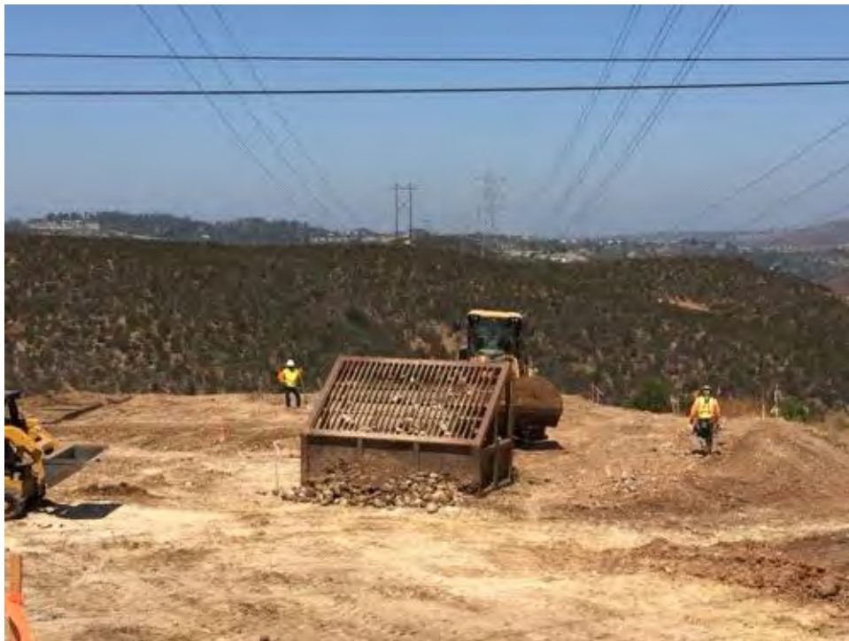
Caption Separator for rock from soil at Pole 03 site .
