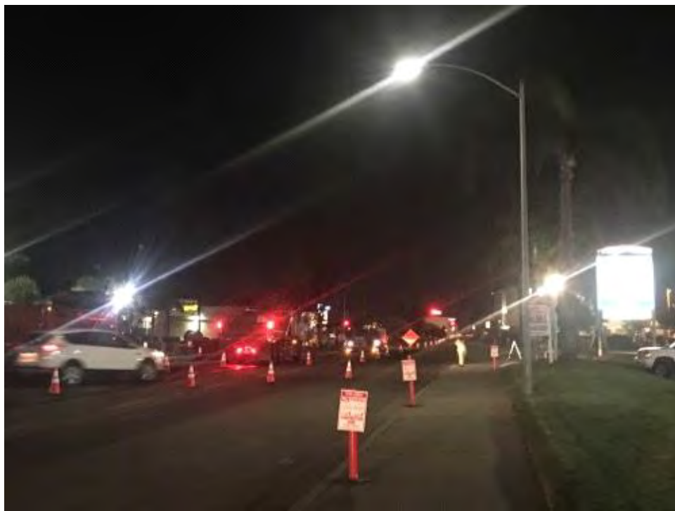
Caption Truck staging and traffic control on southern portion of Black Mountain Road.
