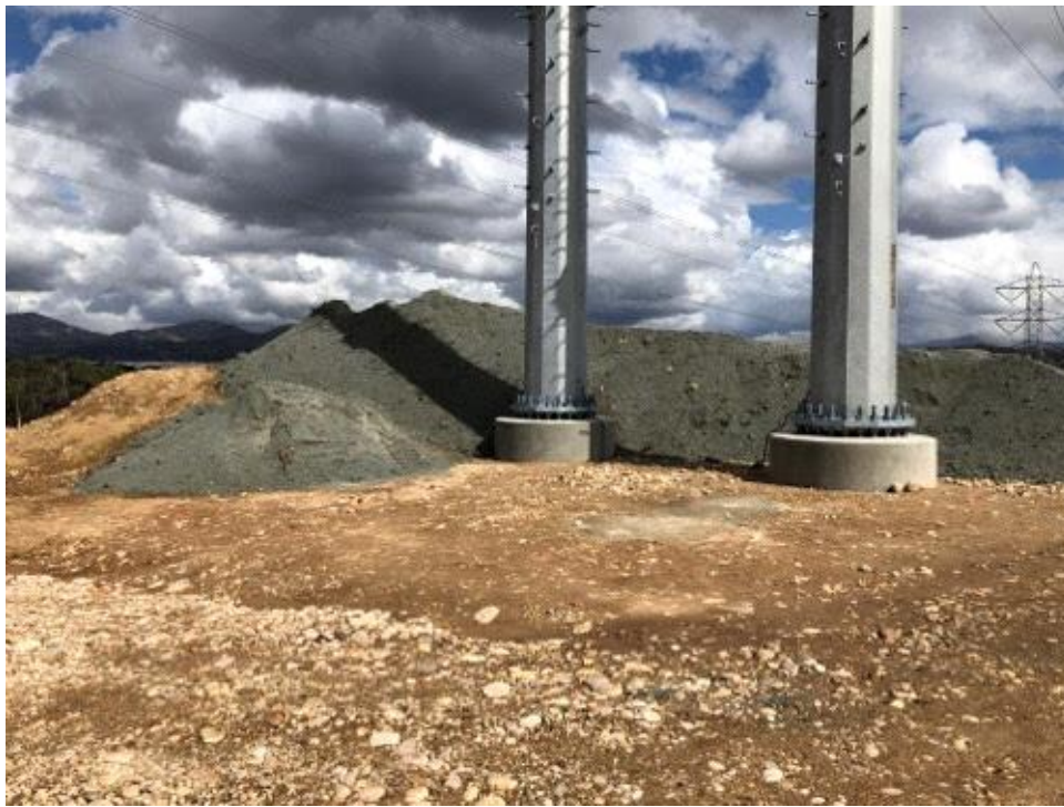
Caption Stockpiles uncovered at P06.
