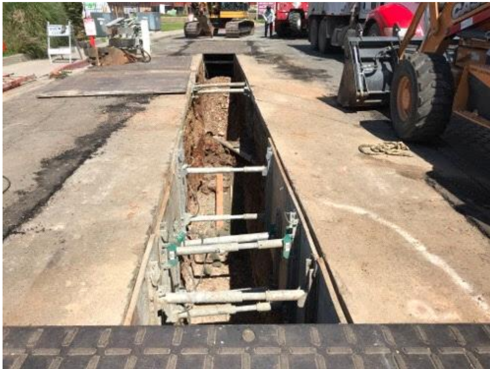
Caption Kearney Mesa Road trench being excavated with vacuum truck due to existing electric utility.
