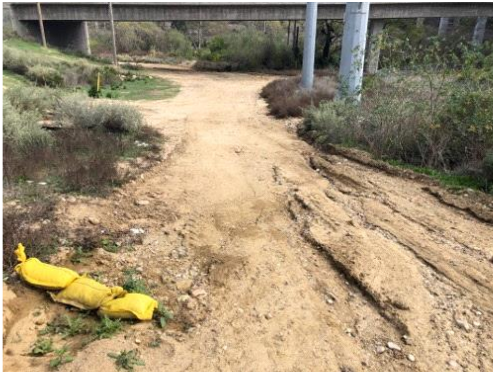
Caption Water rilling on road west of CC MM CP.
