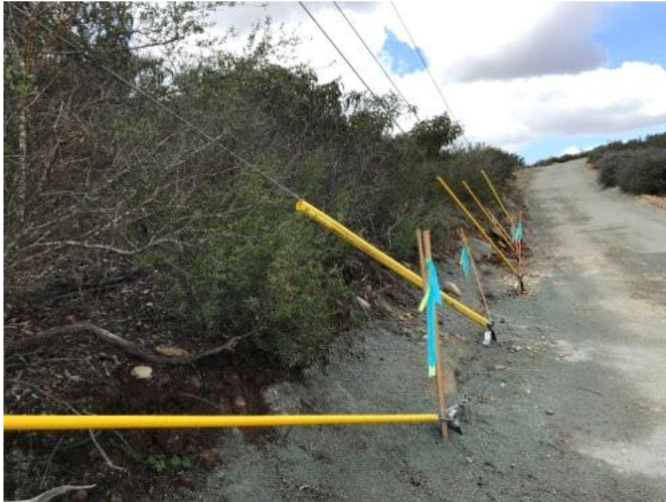
Caption Anchor wires for P05.
