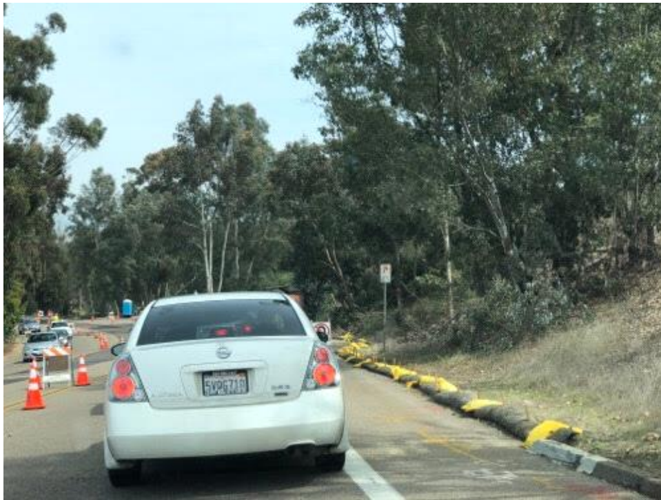
Caption Pomerado Road traffic control and BMPs.
