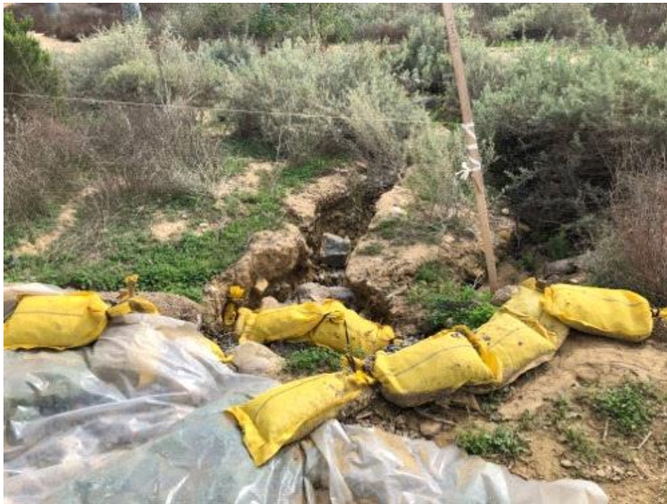
Caption Incised channel west of culvert outlet CC MM CP.
