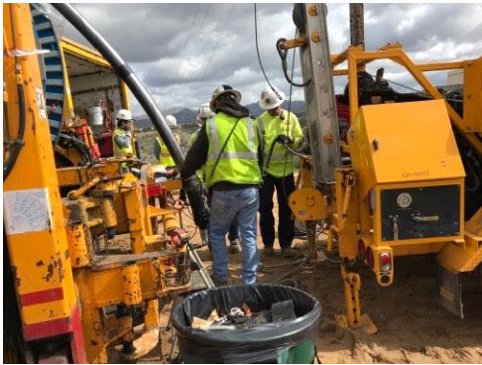
Crew getting ready to pull the cable in the vault at P03.
