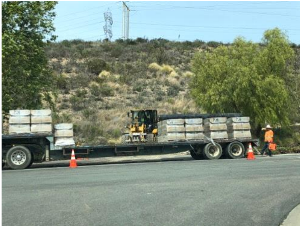
Caption Stone/brick unloading on Stonebridge Parkway for P05. Photo Attributes Capture Date/Time: Mon Mar 12 2018 13:42:19 GMT-0700 (PDT) Coordinates: 32.921689, -117.044177 View Direction: North
