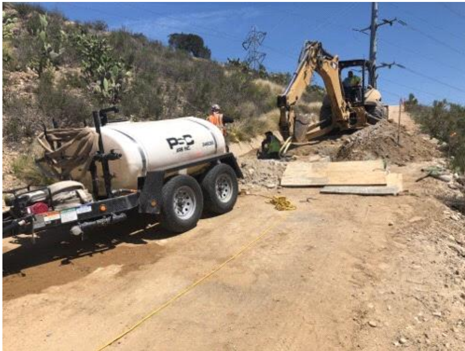
Caption Vault leveling in access road to P05. Note fire equipment on site.
