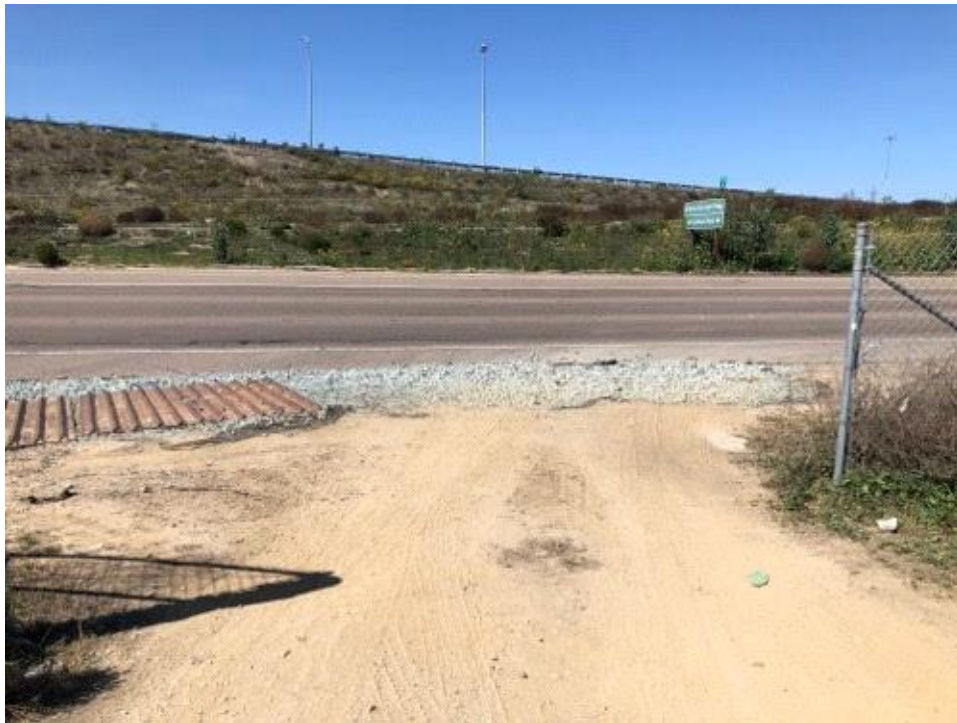
Caption Access gate for staging area north of CC MM CP. Note rumble plates not present at gate entrance. Plates are aligned for adjacent fenced storage area.
