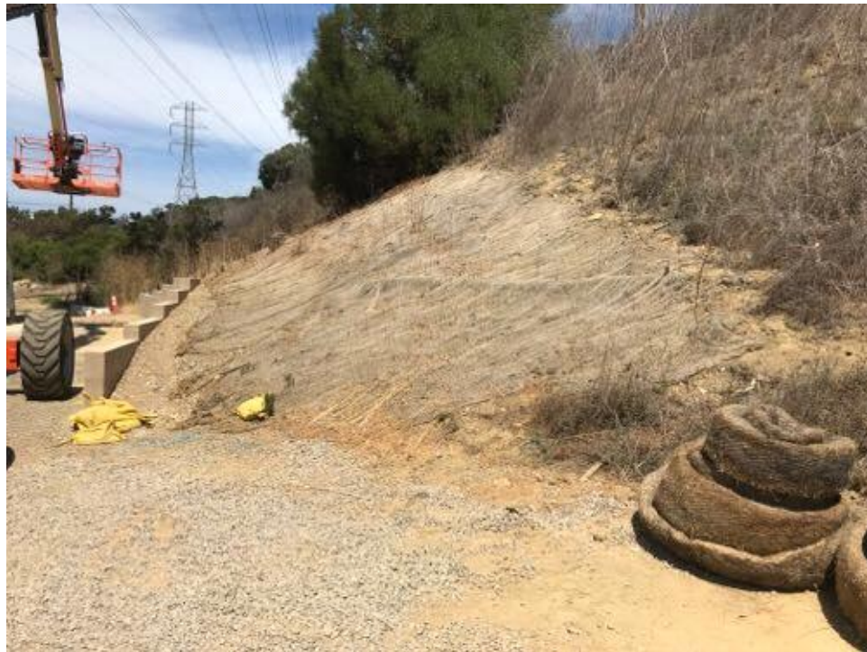
Caption CC MM CP site. Jute netting to be removed and area will be hand seeded and hydromulched on Sept 5.
