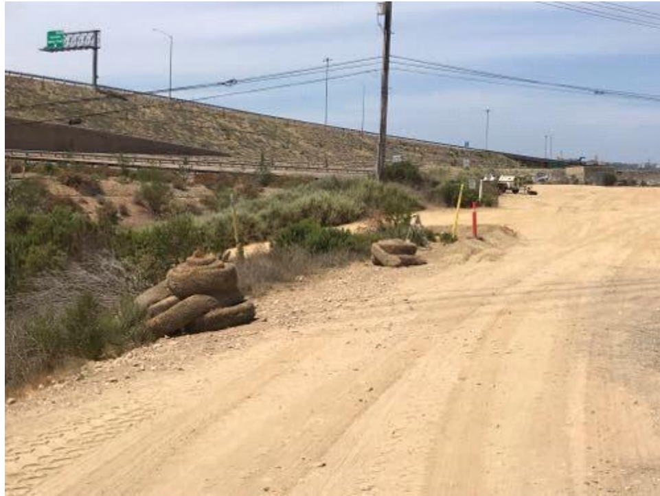
Caption Fiber rolls are ready for removal at CC MM CP site.
