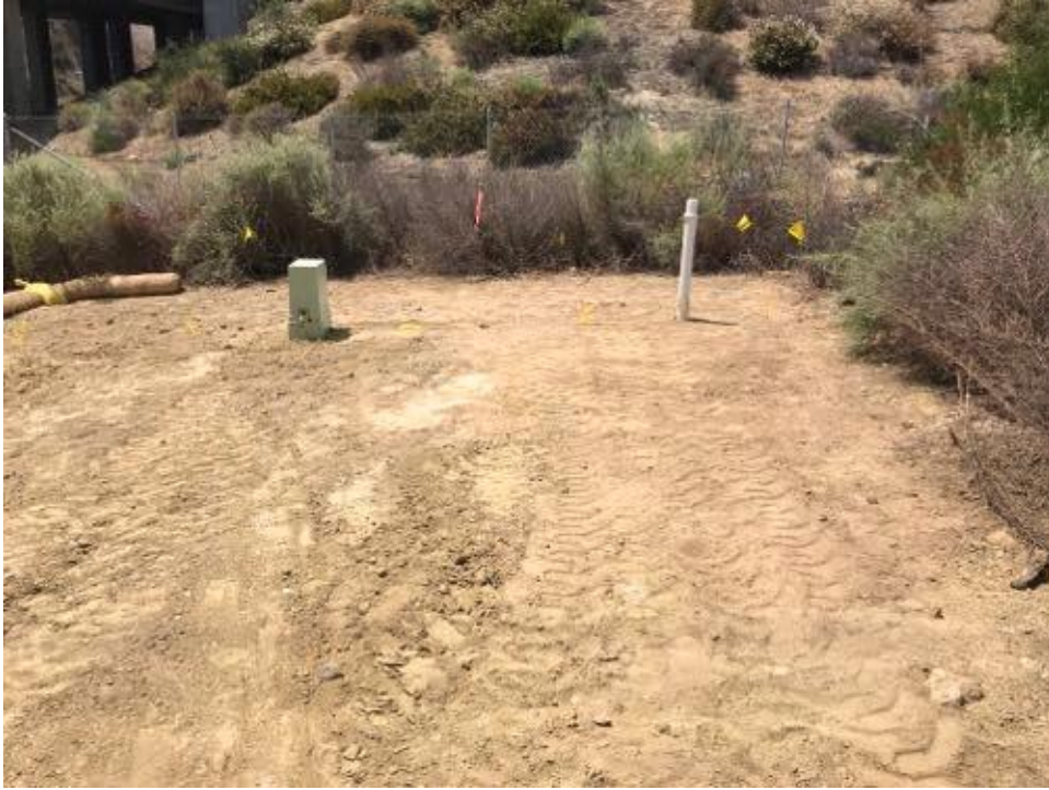
Caption KM 04 AC mitigation site for Kinder Morgan gas line at CC MM CP location. Area will be seeded and hydromulched on Sept 5. Apparatuses are for cathodic protection.
