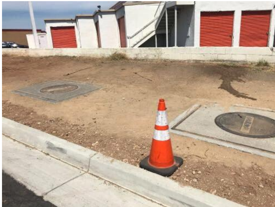
Caption Vault 62 at west side of bore pit will be sodded with grass.
