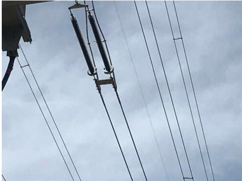
Caption Corona rings installed at CC MM CP.
