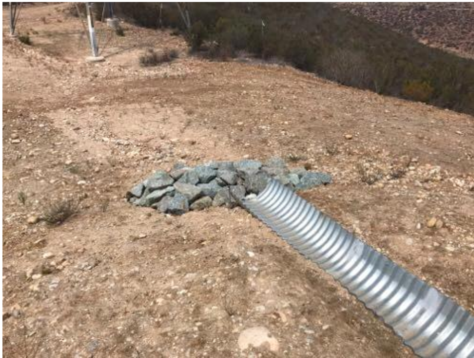
Caption McCarthy drain at P04 still needing modification to prevent downslope erosion.
