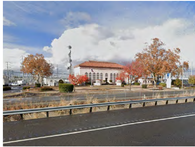
Vaca Dixon Substation
